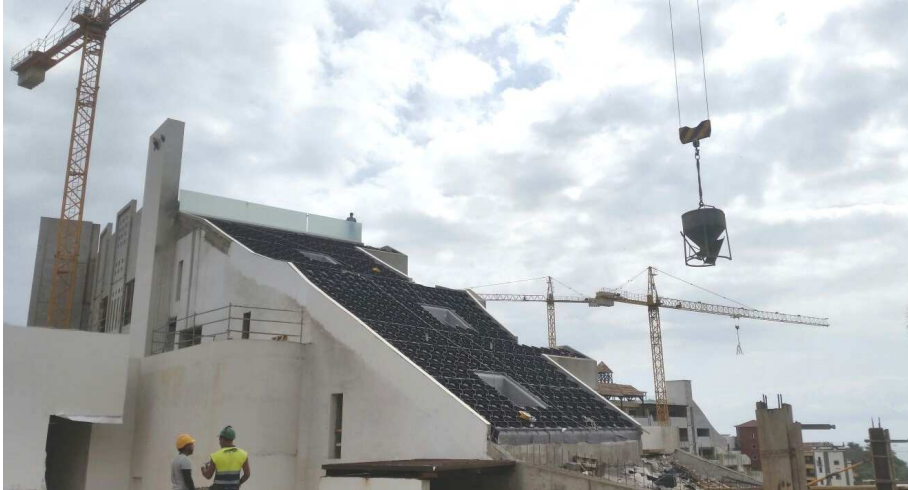
View upon one of the three steep pitched roofs after the installation of shear barriers and Georaster.
